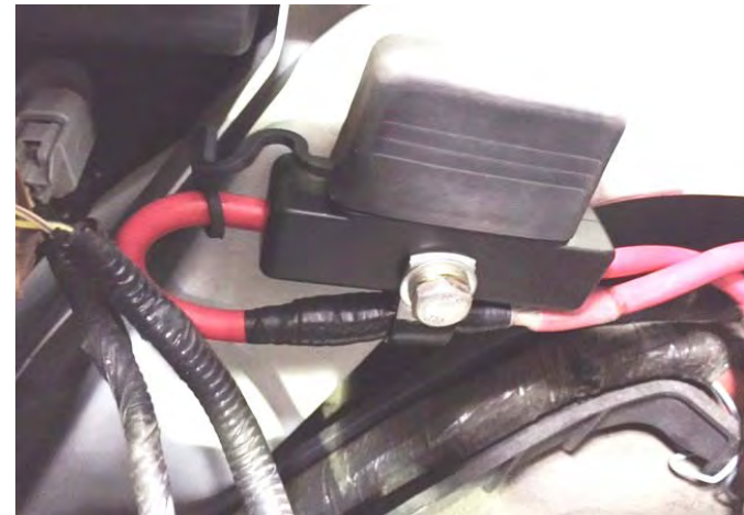
Maxi Fuse shown properly secured to vehicle with bolt and clamp.
